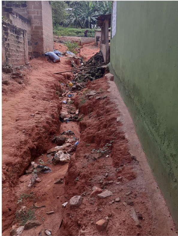
Fig. 9 Road erosion caused by surface runoff in hilly parts of Pokuase. Source: authors' fieldwork, 2019
