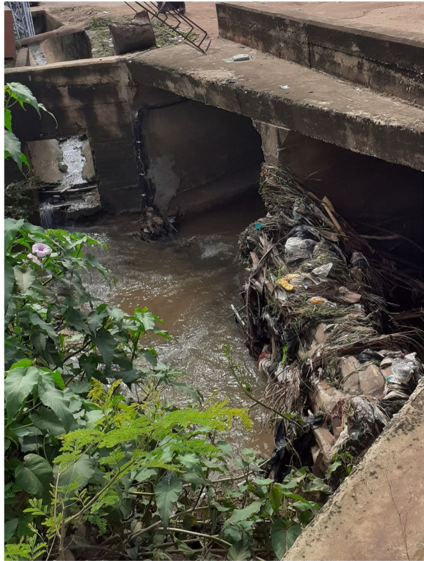
Fig. 6 Waste blocking a culvert in Santa Maria. Source: authors' fieldwork, 2019
