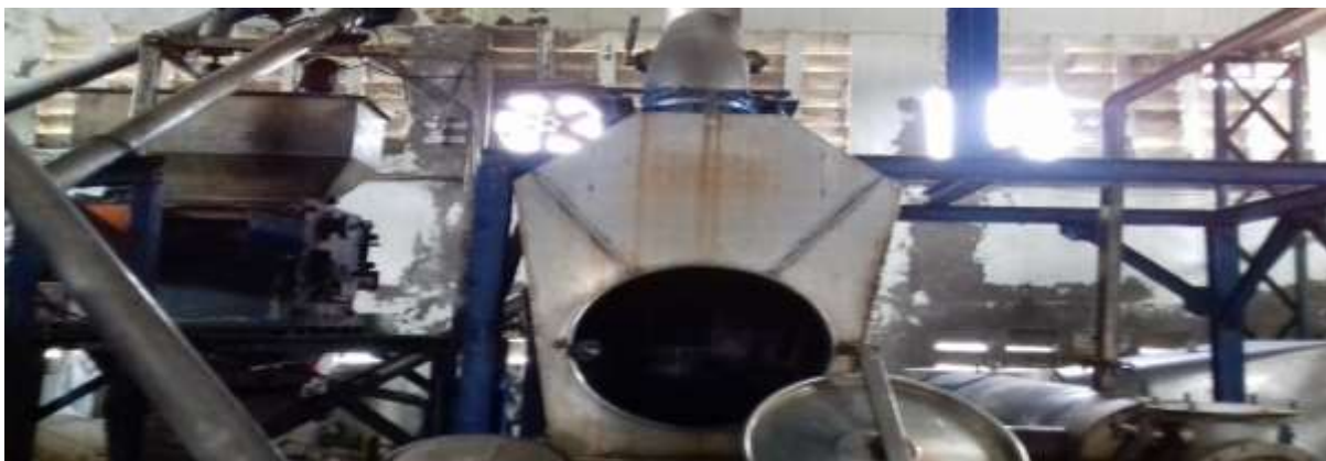
Figure 3.1. 6: A dryer for drying the refined salt (it has heat exchange column).
