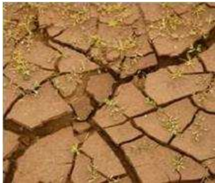
(c) Shrinkage cracks of expansive clays
