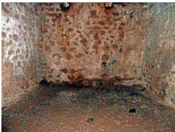
Figure 3. Section of the male slave dungeon, Cape Coast Castle. Photograph by author.
