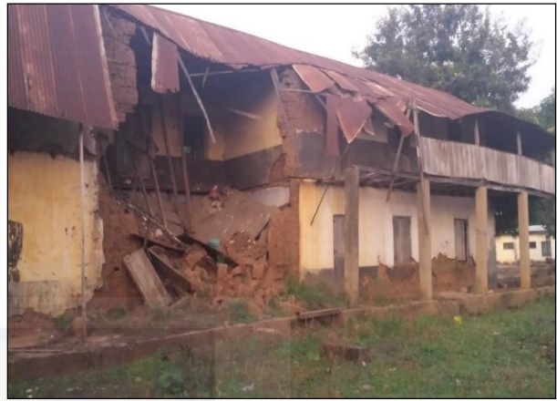
Figure 2: collapsed court house
