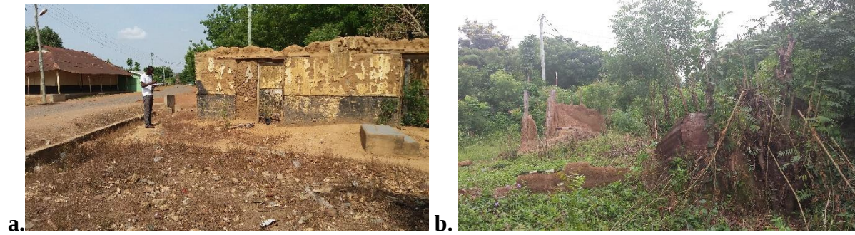
Figure 64a: collapsed story building
