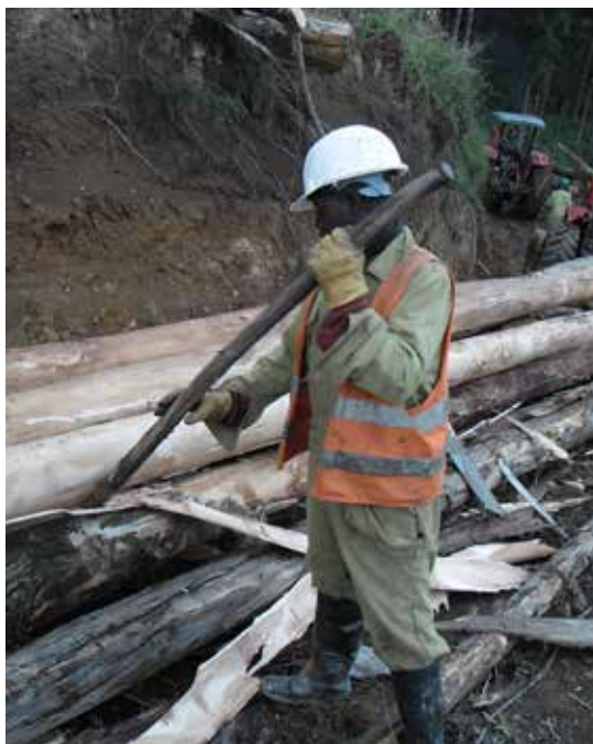
PHOTO 23 Heavy work causing fatigue, heat stress and possibly accidents. Worker adequately equipped.
