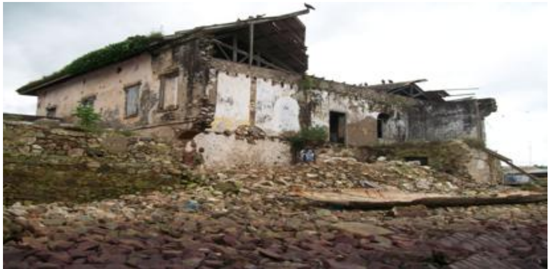
Plate 8.4. This dilapidated one storied structure is reputed to be the oldest European styled house at Dixcove (Picture: Fritz Biveridge).
