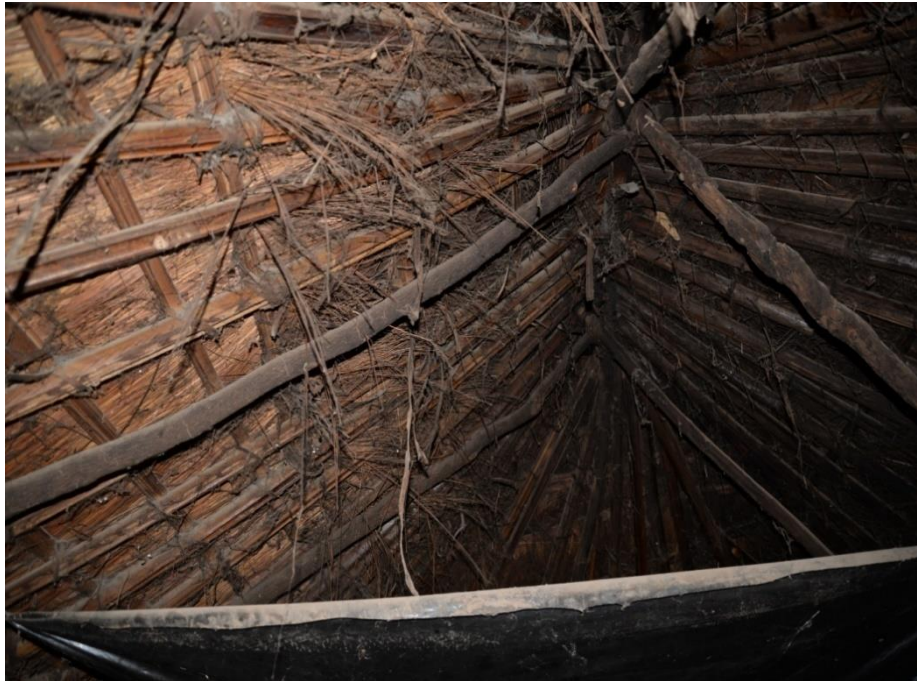
Fig. 4.11: Conical roof framework showing both the kakube and kadeba poles (by D. Genequand)
