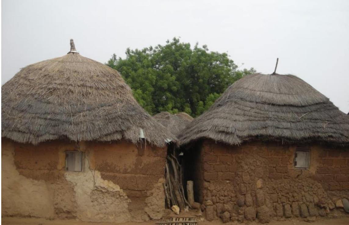
Fig. 4.1: Daub (left) and mud-brick (right) rectangular buildings (single rooms) with conical thatch roof in House 8 (by D. Genequand, 2016)
