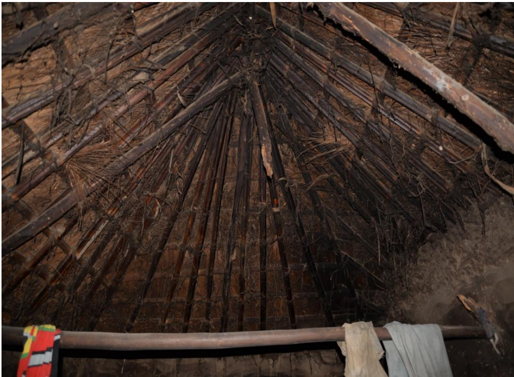
Fig. 4.14: Roofing framework for Type 1B showing the central rafter and broken rafter from the apex (by D. Genequand)
