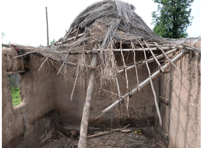
Fig. 4.17: Collapsed building showing the square-like frames of the framework (Photo by D. Genequand)
