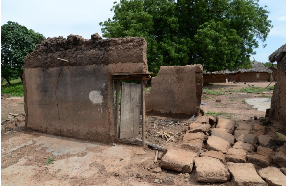
Fig. 5.10: Abandoned building undergoing disintegration (Photo by D. Genequand)
