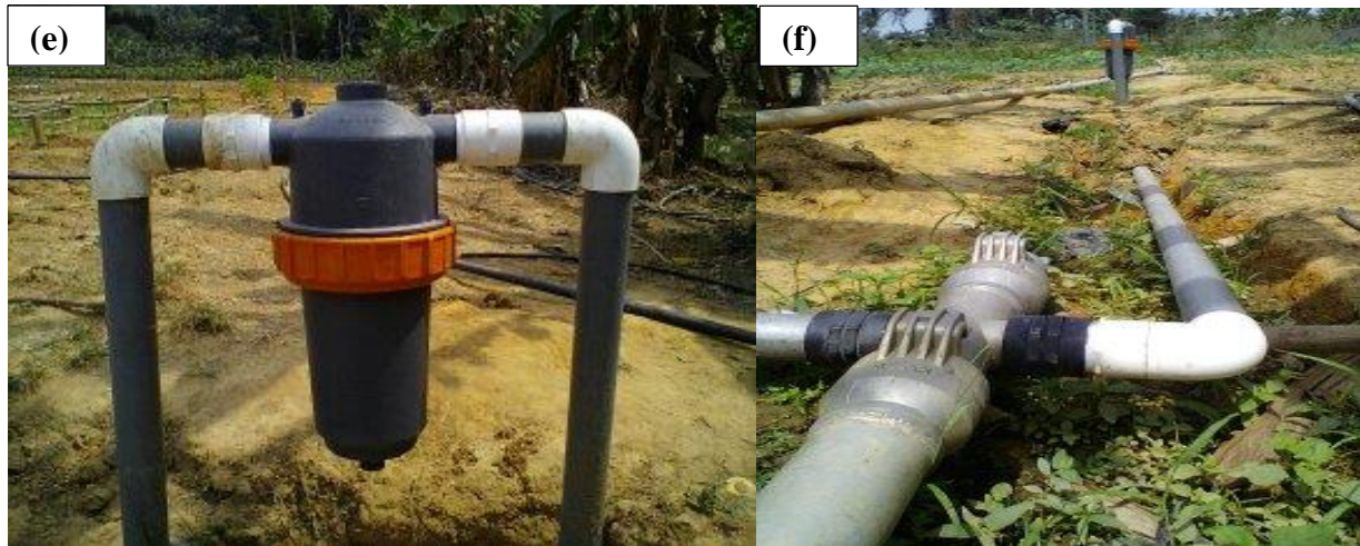
Figure E3. (e) Filter connected to main line and (f) Main line connected to water source (dam)
