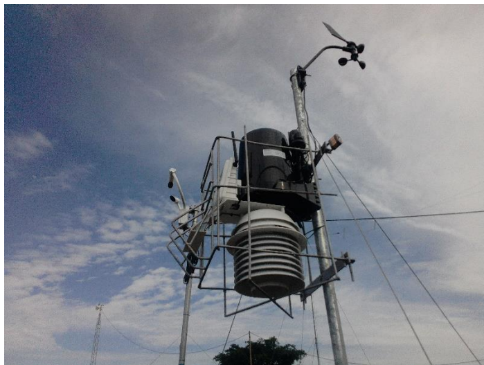
Figure 4.14: Installed Vantage Pro 2 weather station at the Tamale site
