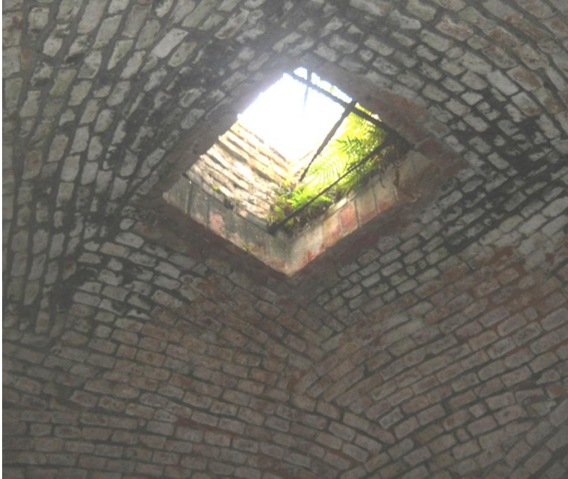
Figure 10 Photo of one of the three ventilations of the dungeon of fort Gross Fredericksburg (Photo by E. A. Nyarko, 2012)
