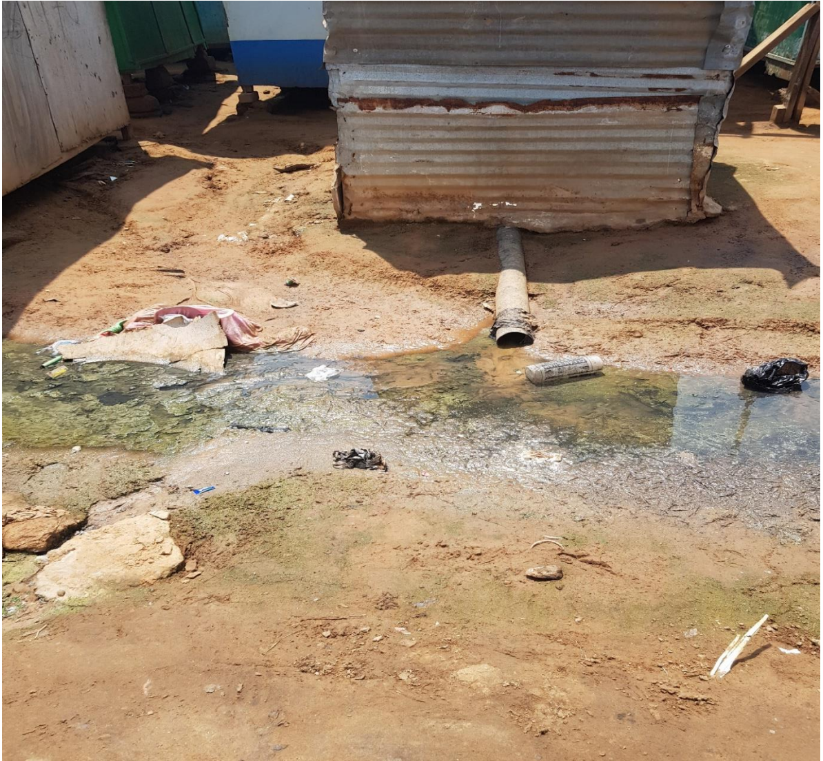
Plate 4.2: Greywater connection on bare ground in informal settlements, Ogbojo
