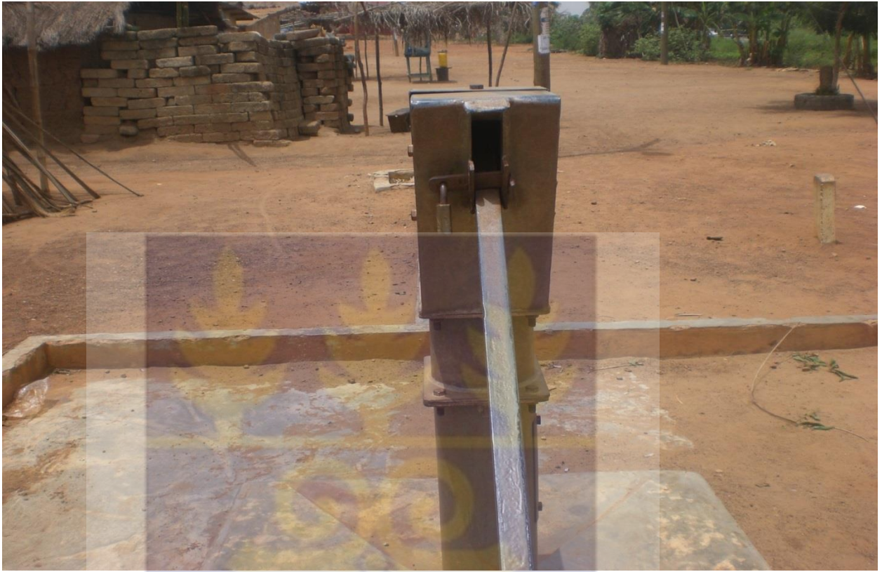
Plate 4.2: Spoilt mechanized borehole at Ekumfi Swedru
