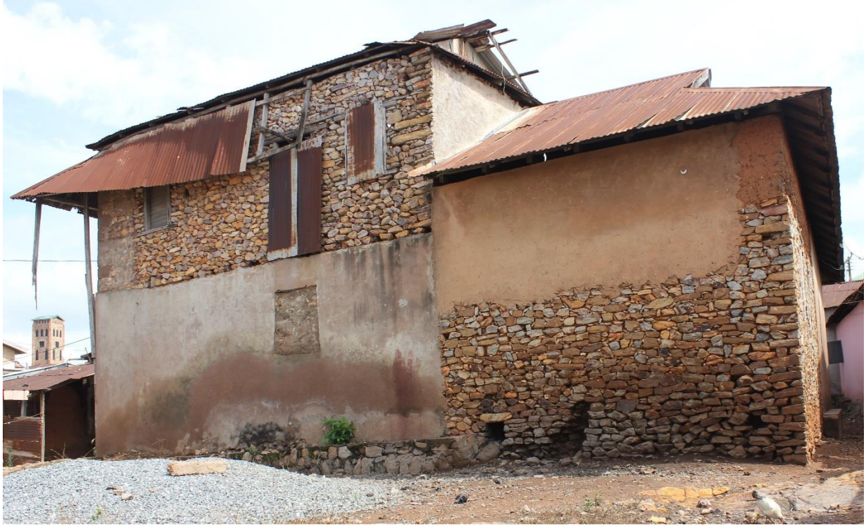
Figure 3.3 Picture of a house built with stones at Larteh. (Photo credit: Author's collections).
