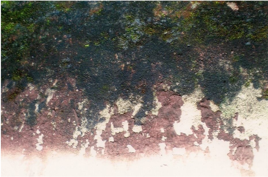
Figure 1: Plate 10 (A freshly degraded emulsion painting (infected wall))
