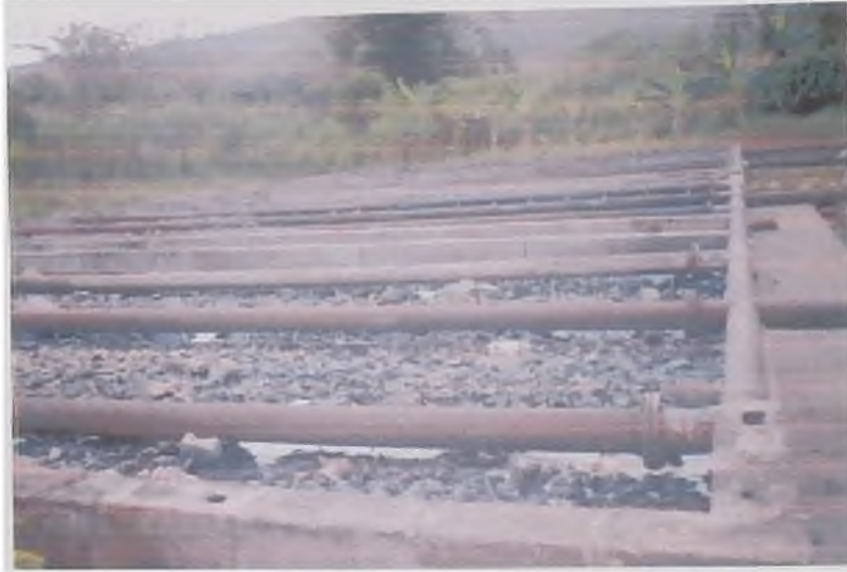
Plate 10 Part of the ATL Treatment Plant showing perforated pipes on filter bed.
