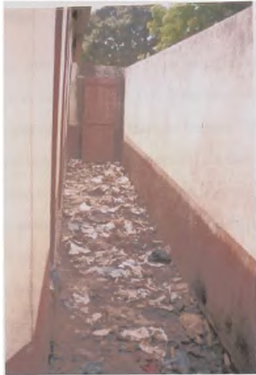
Plate 6 Entrance to a Female Public Toilet at New Powmu (Note the filth).
