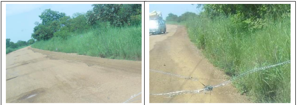
Fig. 5.5 Potholes on the Bolgatanga-Bawku Road
