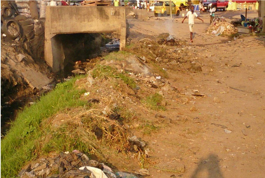
Plate 2: Indiscriminate Waste Dumping resulting in Choking of Storm Drain by Solid Waste in Kasoa Township
