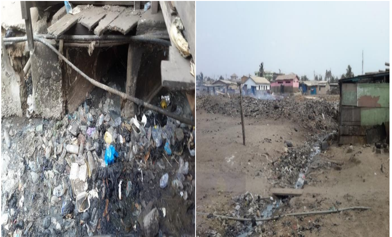
Plate 3. 1 Pipelines found in drains in Chorkor
