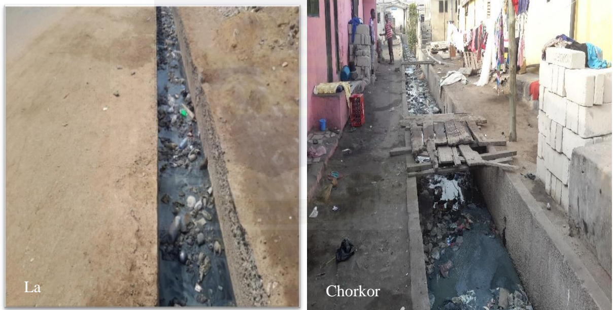
Plate 3. 4 Uncovered Choked Drains within the Communities
