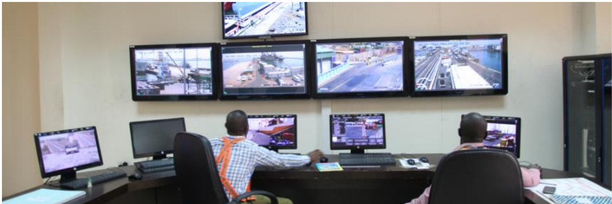
Figure 5.3: CCTV Monitoring Room
