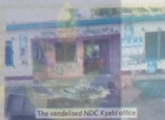
The vandalised NDC Kyebi office
