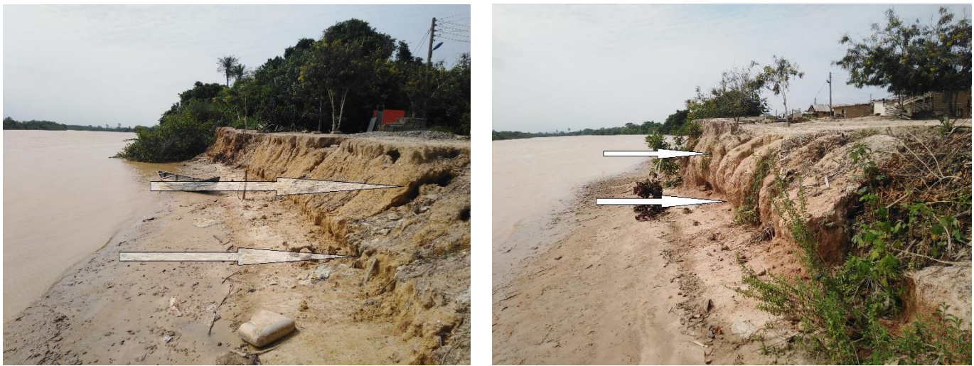
Figure 4.5: Riverbank Erosion at Krobo and Bosomdo.
