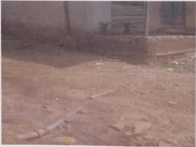
Fig. 5. Penetration of contaminated water into distribution mains
