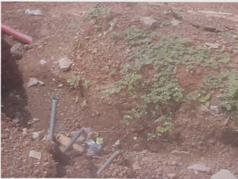
Fig. 7. Contamination of chlorinated water through back-siphoning
