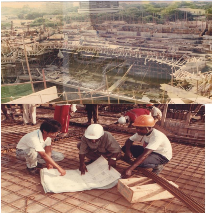
Fig 18: The National Theatre when it was being constructed in 1990. Source: The Estate Department.
