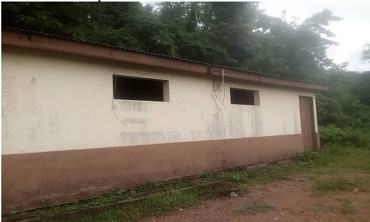
Plate 4. 4 : Detoraited public toilet in Domenase
