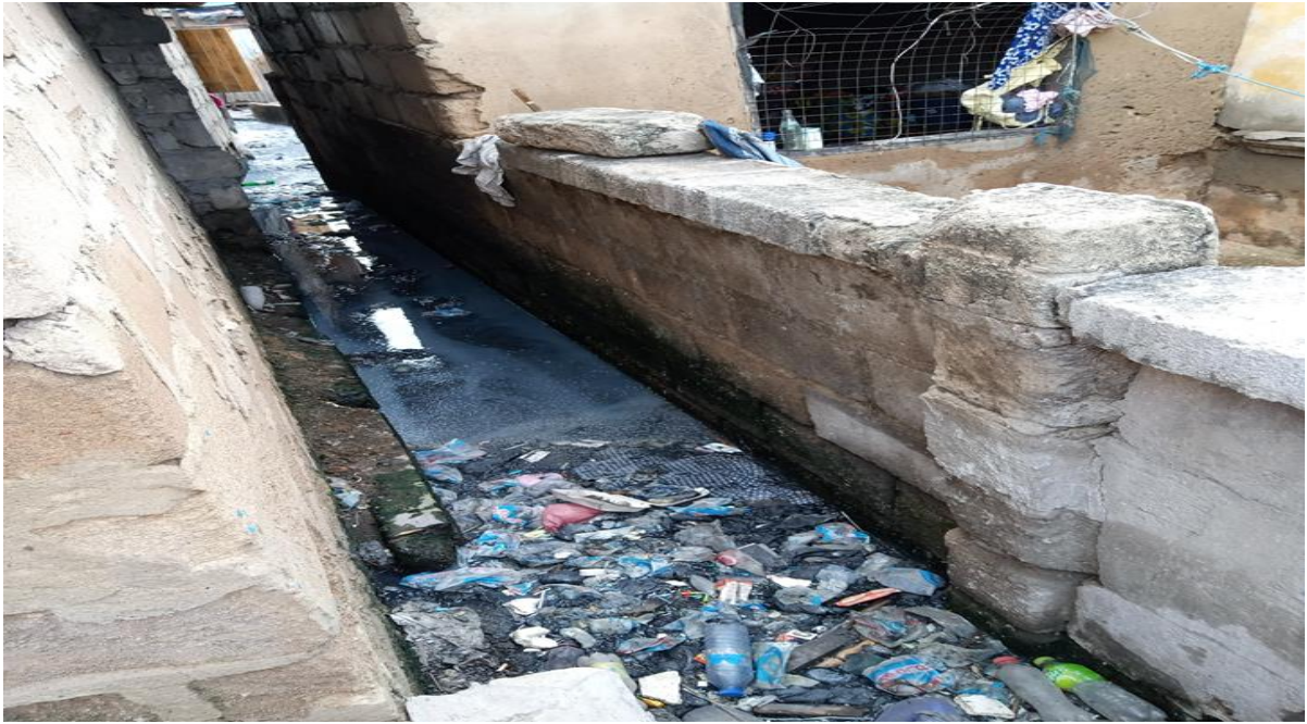
Figure 4.5: Choked gutters within households in Agboglobhie, Accra
