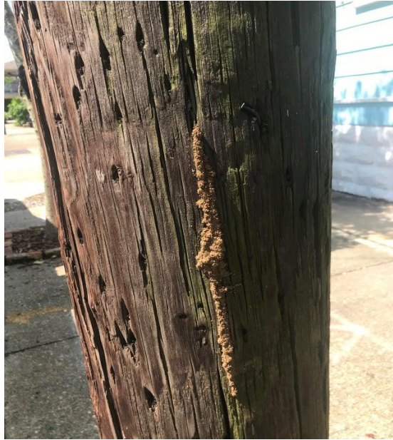
Figure 2.2: Deterioration of timber pole due to ant and termite infestation
