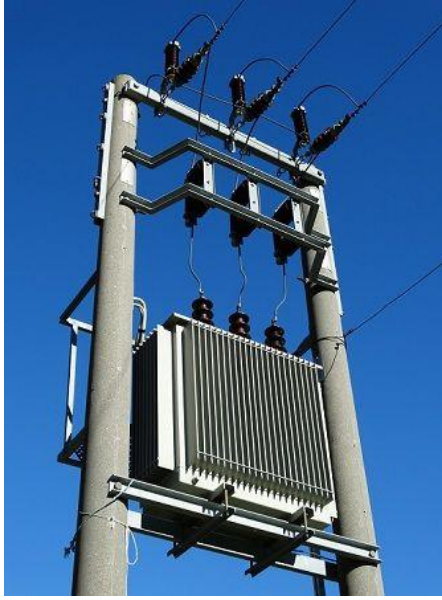
Figure 1.2:High tension pole with mounted transformer
