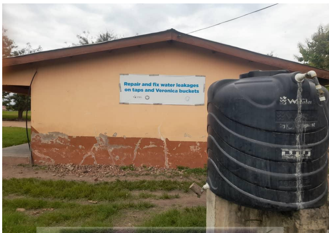
Plate 6: Water storage system in Adaklu Kpodzi basic school in Adaklu District.
