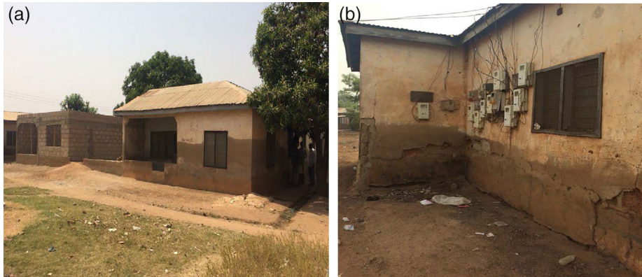
Figure 3. High flood line clearly evident on buildings in study communities.
