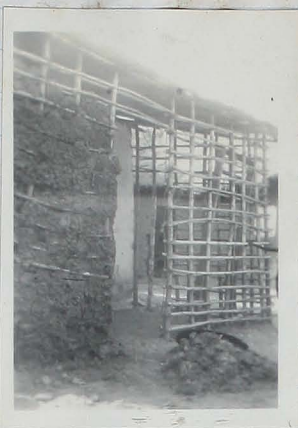
A HOUSE IN BUILDING AT WEIJA VILLAGE SHOWING WOOD FRAMEWORK IN THE WALL.
