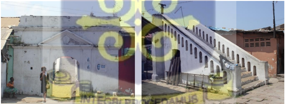
Figure 2.2: Current front view of stairs leading to the upper quarters of the Richter House
