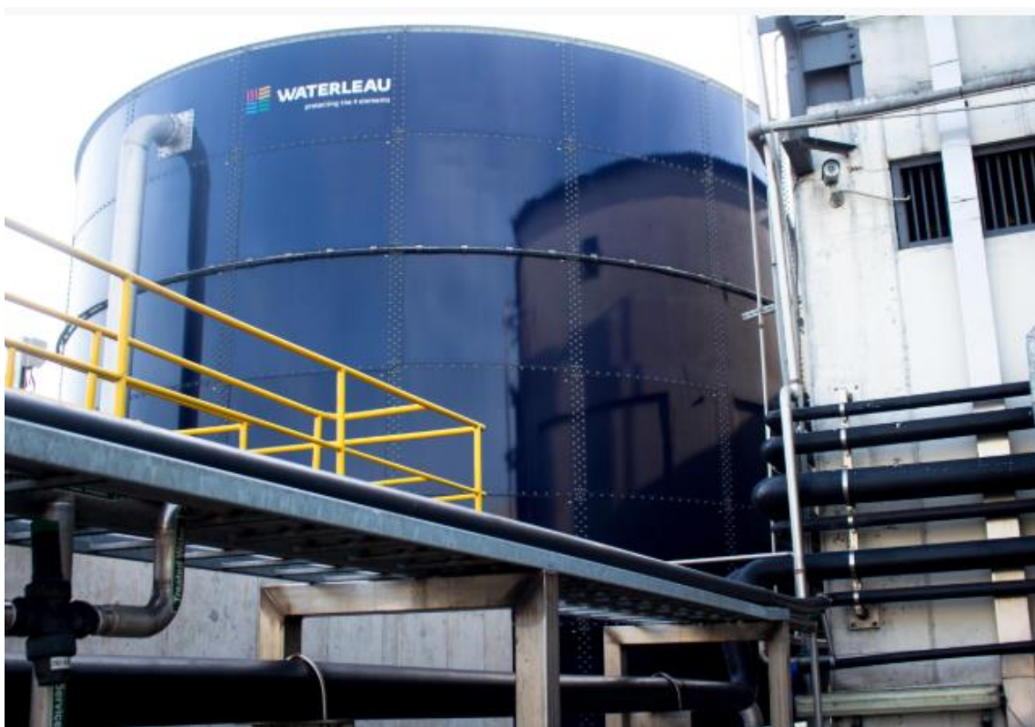
Figure 4.2.4 One of the effluent treatment tanks in ABL
