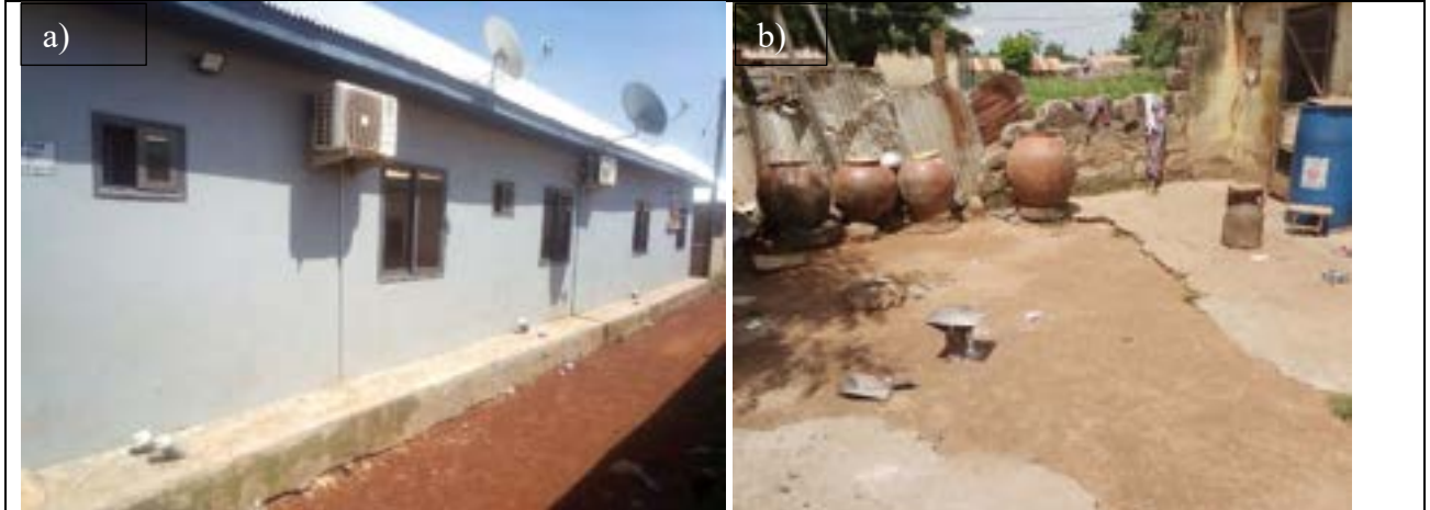
Figure 6.3 Elevated Platforms as a Flood Adaptation Measure a) A building at Kalariga with a well-constructed apron b) A building in Nalung with minimal elevation Source: Field Data, Household Questionnaire Survey, 2023
