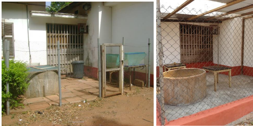
Plate A: Hatchery shed under construction at the Department of Marine and Fisheries Sc., UG
