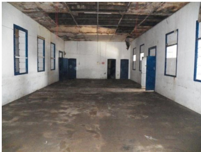
Plate 17: Decay of wooden timber ceiling members (Source: Author)
