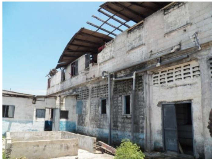
Plate 13: Southern façade showing damaged roof and with broken doors and windows ( Source: Author )
