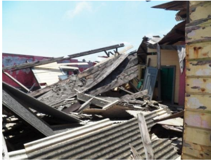
Plate 24: View of the collapsed roof at the South-western part of the building
