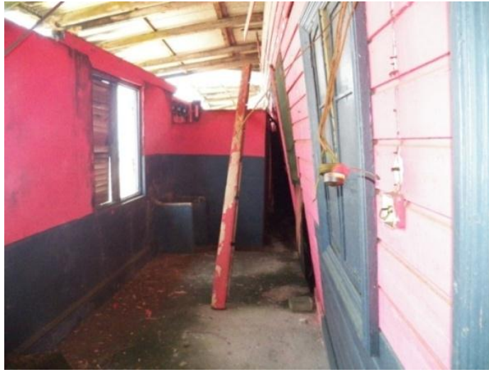
Plate 22: Collapsed timber partition; concrete slab introduced on top of wooden first floor slab ( Source: Author )
