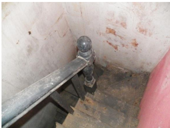
Plate 19: Broken wooden stairs to the upper level ( Source: Author )
