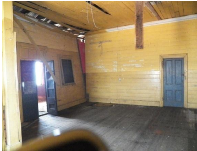
Plate 20: Skewed timber partitions and damaged ceiling on the first floor (Source: Author)
