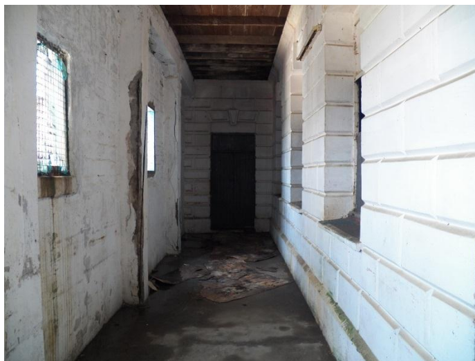
Plate 11: Masonry block work on the ground floor displaying craftsmanship of that period ( Source: Author )
