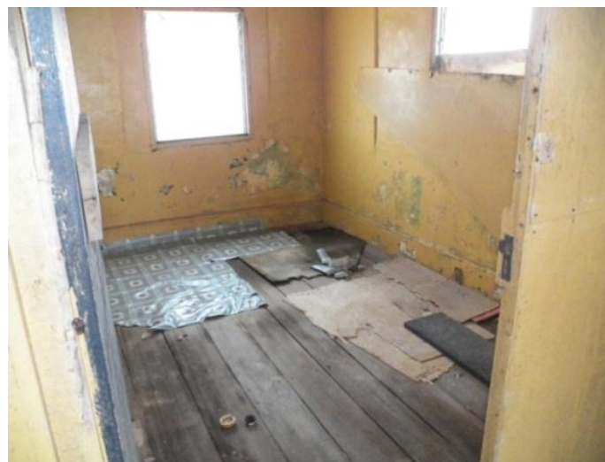
Plate 21: Damaged timber flooring covered with loose plywood boards (Source: Author)
