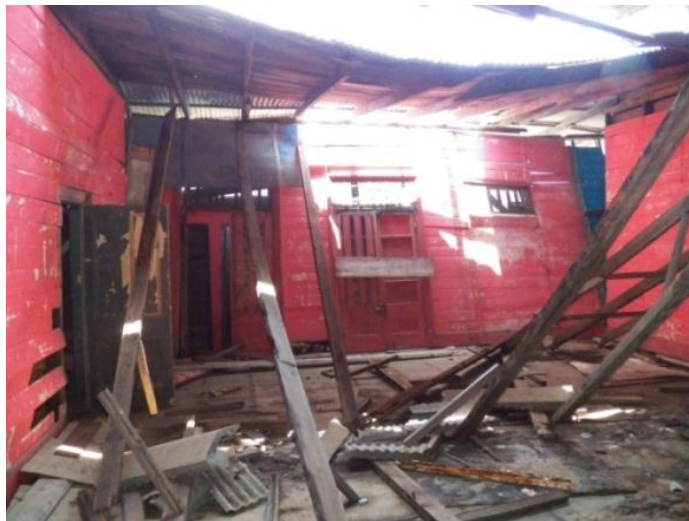
Plate 23: Caved in roof on the first floor ( Source: Author )
