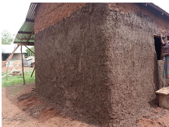
Fig. 2 It is the responsibility of women to plaster a newly constructed earthen building in Tamale (Source: the authors, taken in 2022)
