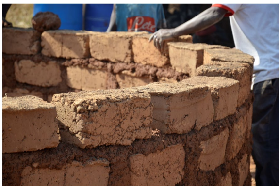
Fig. 4 A man demonstrating the construction of a building using sundried earth bricks and earth mortar joints in Wa (Source: the authors, taken in 2021)
