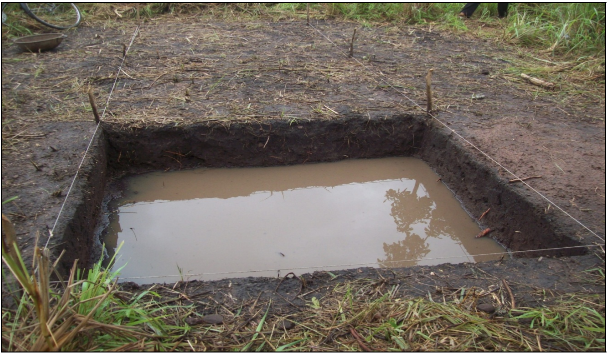
Figure 5: Trench Filled With Rain Water.
