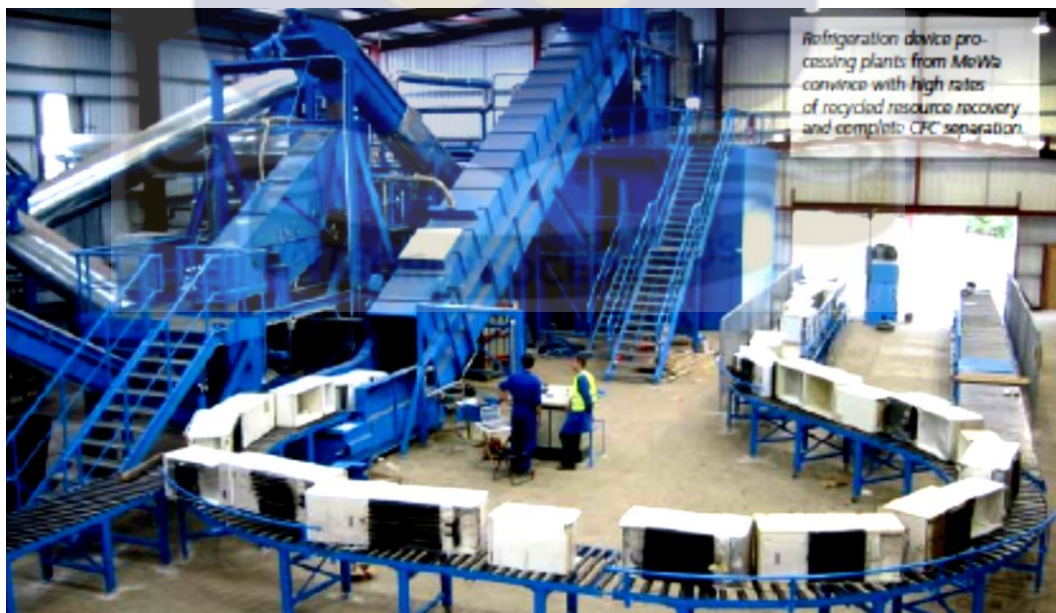
Figure 2.4: A stage 2 refrigerator processing plant in operation
