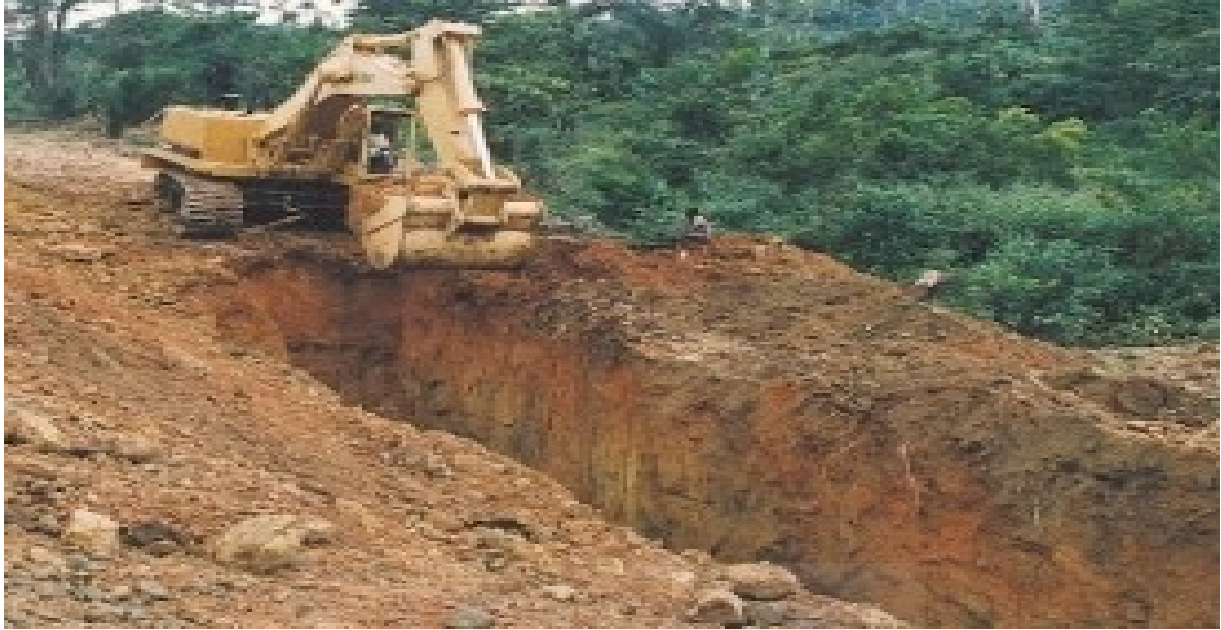
Fig. 3.1.2 showing mechanical excavation of TKBB001 in the North West _South East Direction
