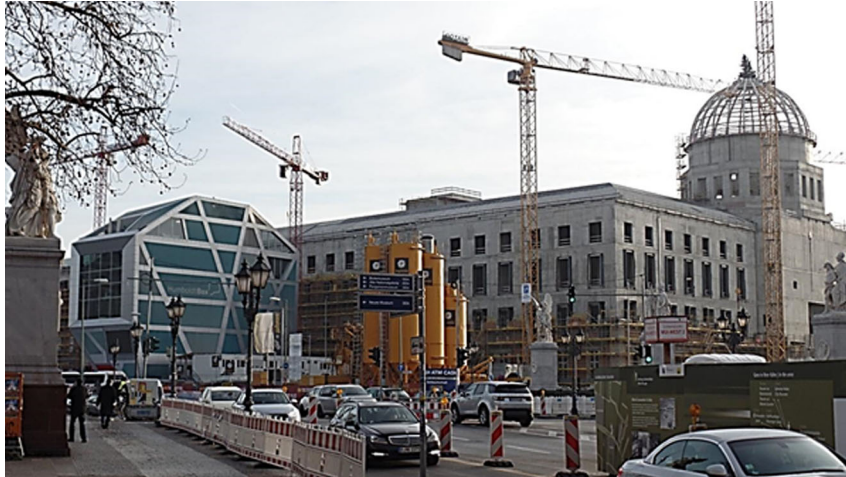
Figure 3. Ongoing construction at the site of the Humboldt Forum in Berlin. The “Humboldt Box” is visible in the front, and the reconstructed City Palace is in the back. (Photo by the Author) [This figure appears in color in the online issue.]
