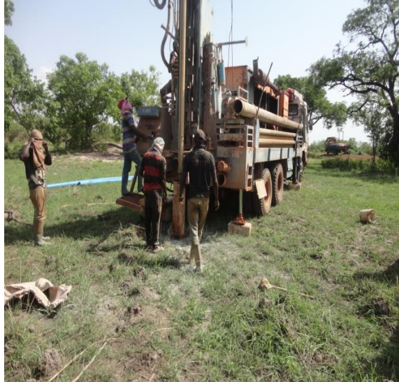
Figure 3-2. Rotary Drilling machine
