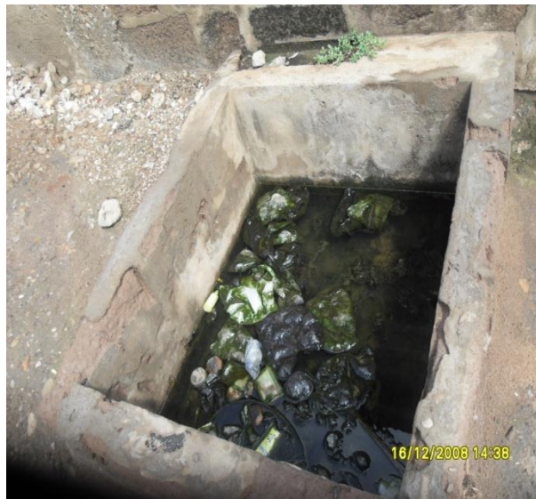
Plate 3.1b Fire Hydrant Used as Point for Store of Waste Water
