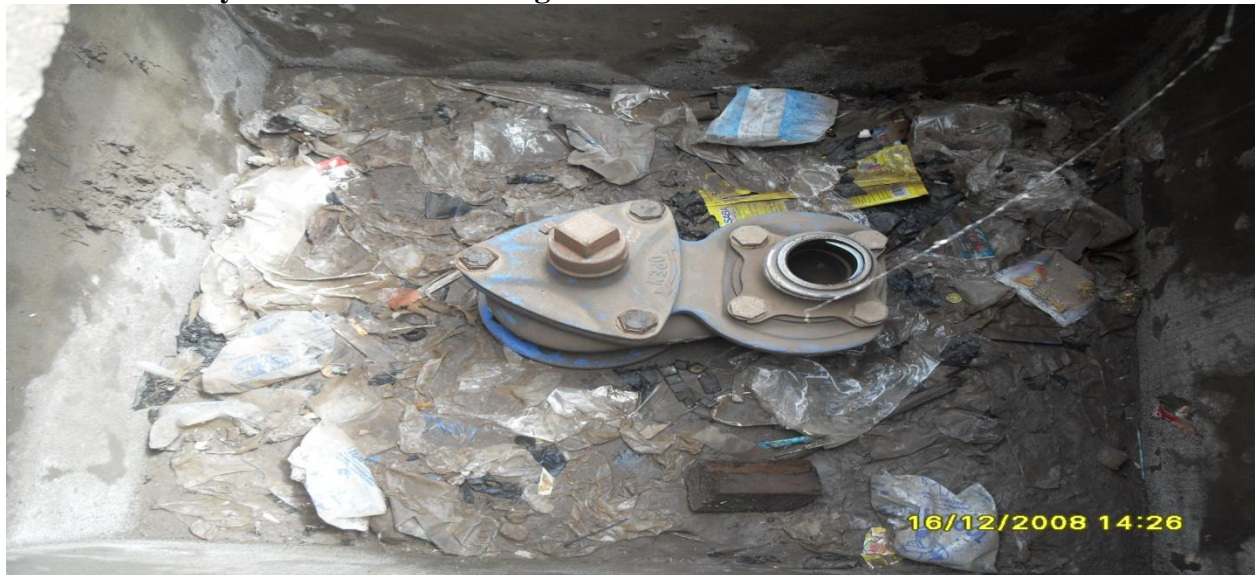
Plate 5.4 Fire Hydrants Used as Garbage Collection Points
