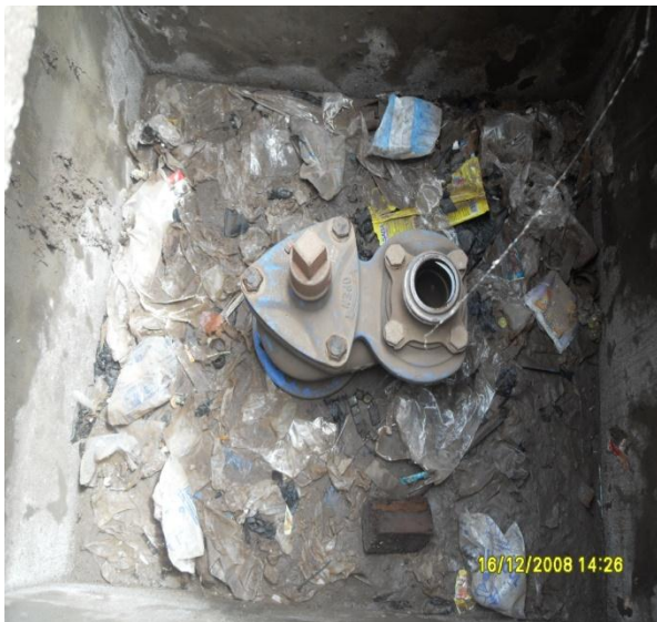
Plate 3.1a Fire Hydrant used as Garbage Collection Point
