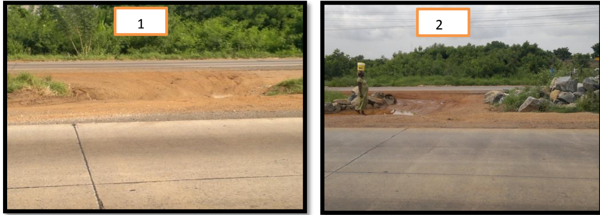
Figure 4.10: Illegal U-Turns on the Accra-Tema Motorway
