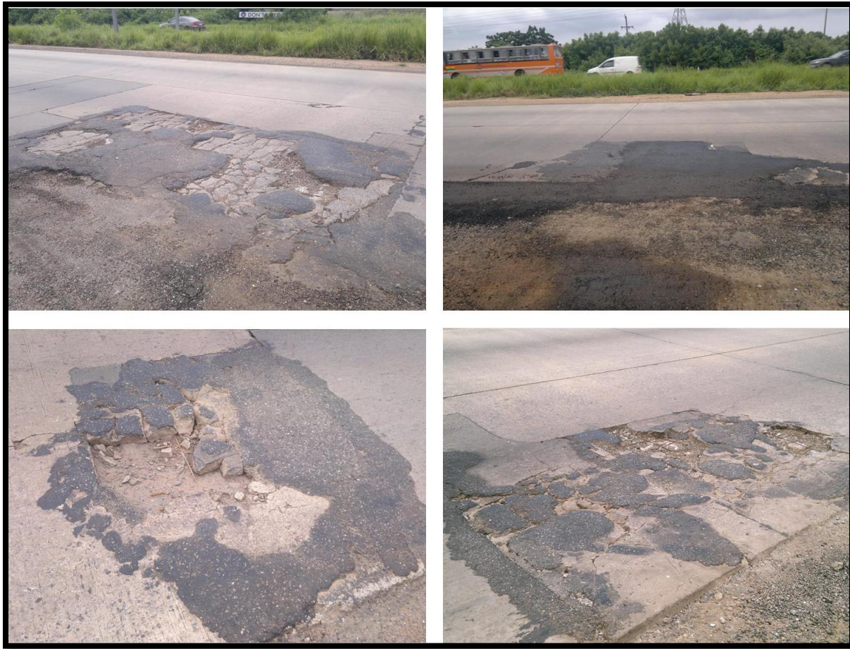
Figure 4.19: Sampled Potholes and Cracks on the Accra-Tema Motorway
