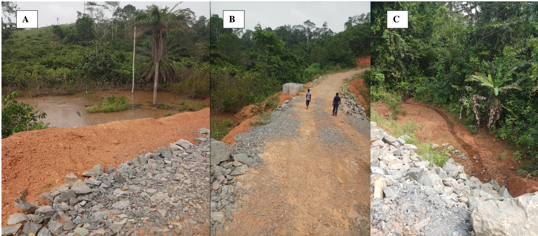
Plate 4.4 River Dammed by a Road
