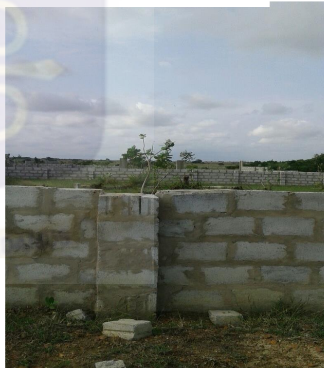
Plate 5.2. Encroaching Portion of the land at the site with a Wall
