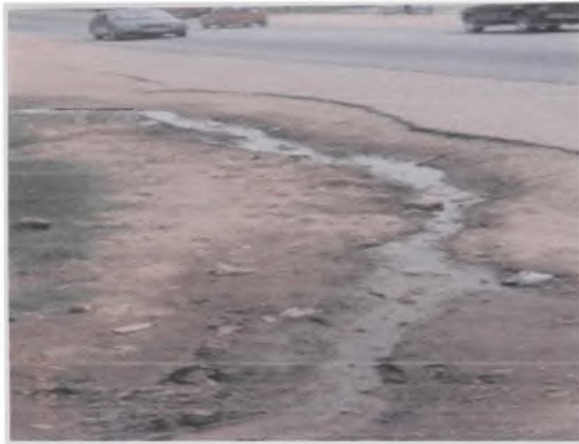
Plate 5: Sample collection site at Achimota. A narrow stretched pool of water flowing from a leaking water supply pipe and exposed to sunlight.
