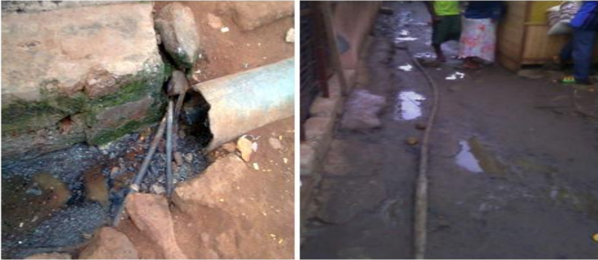
Plate 4.3: Pipelines located on the surface ground
