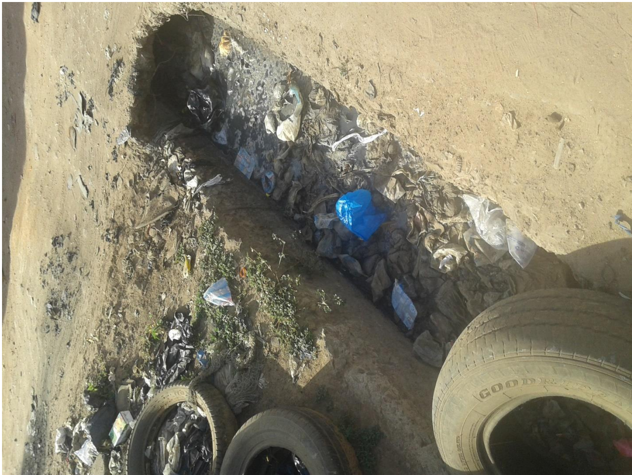
Plate 3. 3: A rubbish filled gutter
