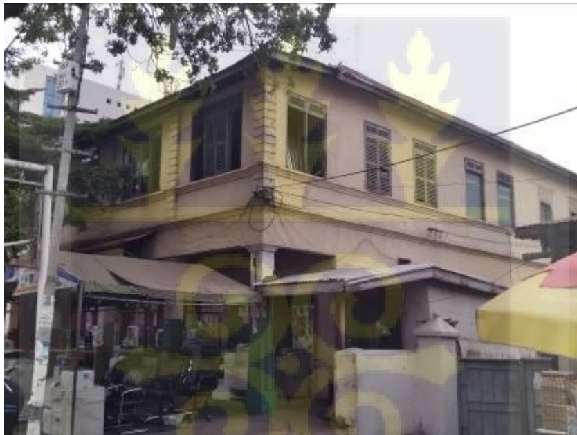
Figure 4.10: Dilapidated Old Building in Adabraka Community
