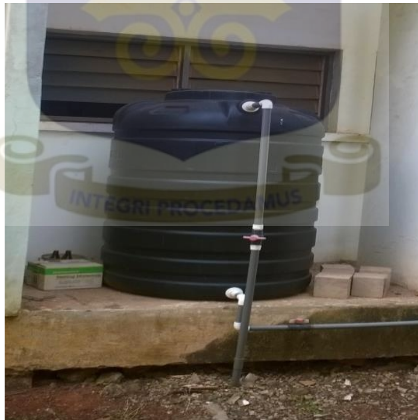
Figure 3. 3: The 1000L PVC water Tank that supplies water to the Flow Rig
